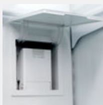
Air Purification System
